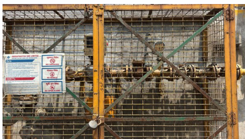
Piped Natural Gas (PNG) installation with Indraprastha Gas Limited safety signage at an industrial unit
