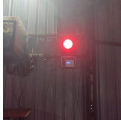
LED indicator showing red — a high-dust alert state at a site
