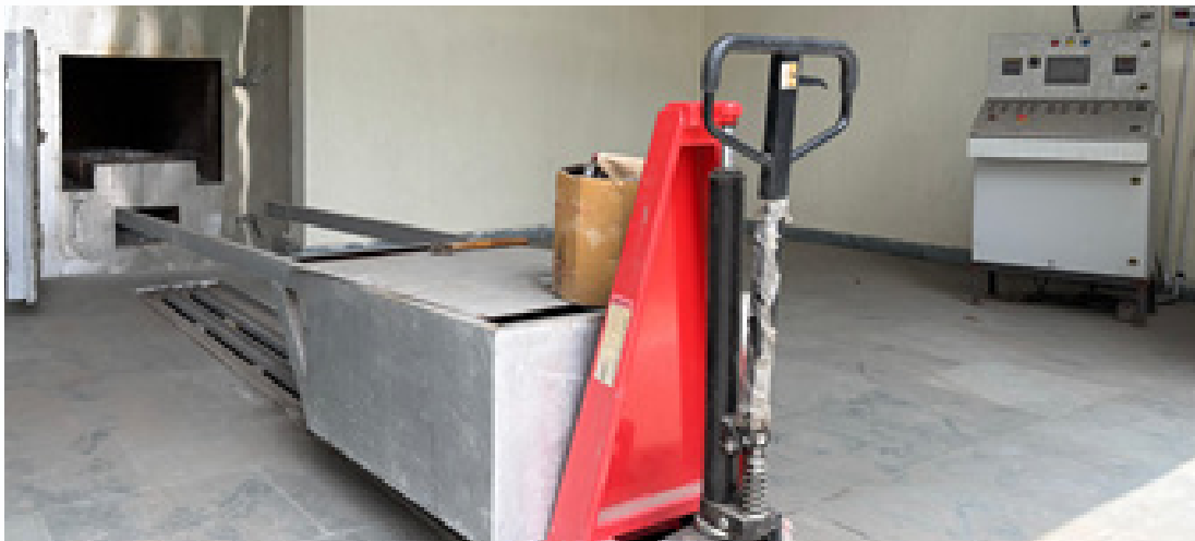
PNG-fired cremation chamber with control panel
