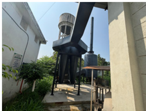
The dual-stage (dry + wet) Air Pollution Control Device
