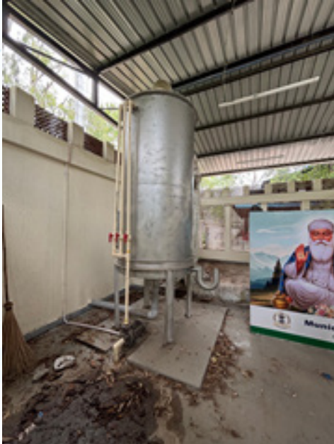
Wet scrubber for flue-gas treatment
