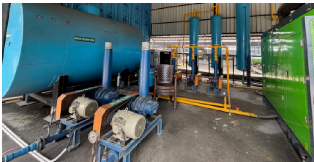
Biogas pressure vessel, blowers, scrubbers and generator at the plant
