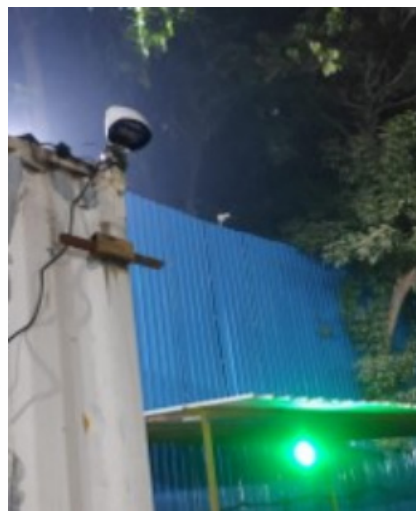
CCTV and LED indicator at a construction site
