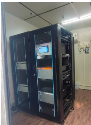
Analyzer racks inside the station: GC-FID (VOC), GC-ECD (sulfur-odour) and FTUV (NH 3 ) units
