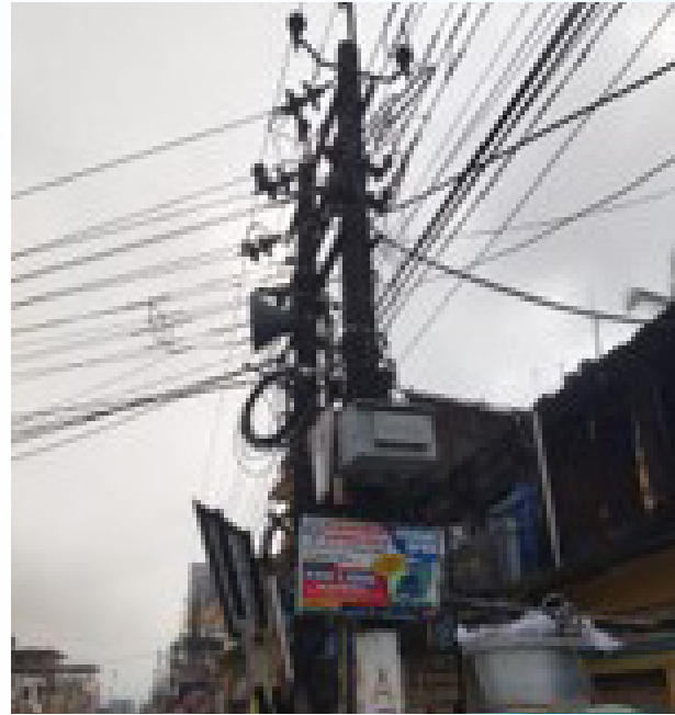
A pole-mounted CCTV camera and public-address unit at a Nalbari market junction
