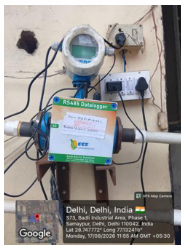
RS485 datalogger transmitting continuous emission data, Badli Industrial Area, Delhi
