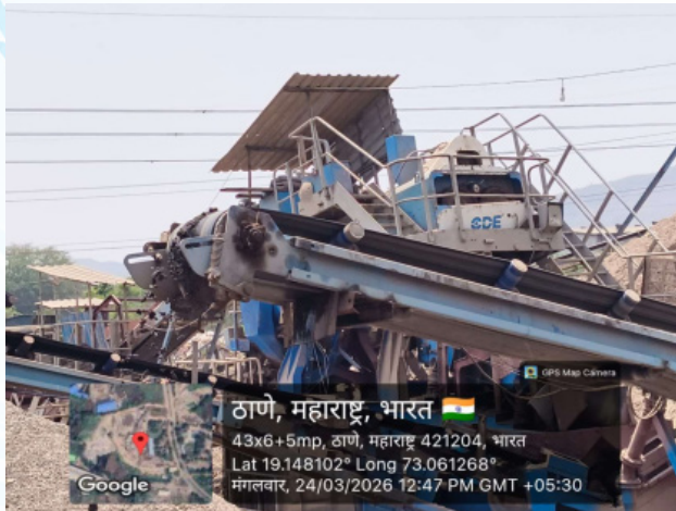
Crushing and conveyor unit at the C&D waste processing facility
