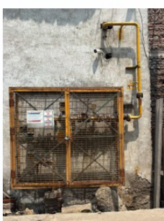
PNG supply line and caged gas installation at an industrial unit, Delhi
