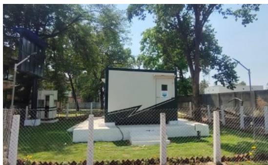
Station shelter within a secured, fenced compound at a major industrial cluster
