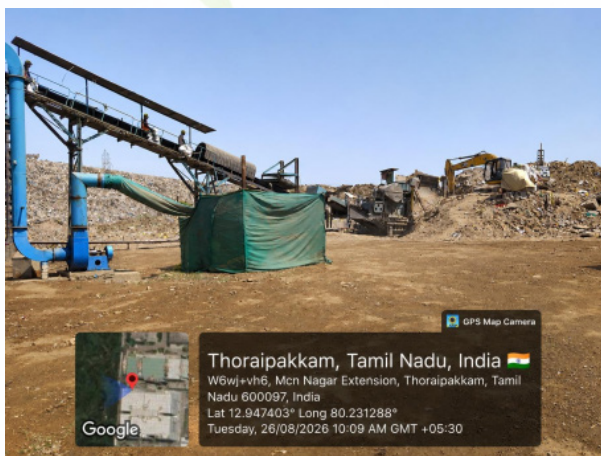
Conveyor, crusher and screening unit processing C&D debris at Thoraipakkam
